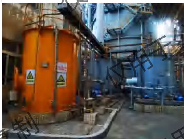
湿式除尘器碱液罐
