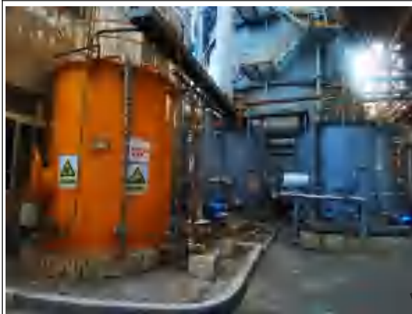
湿式除尘器碱液罐
